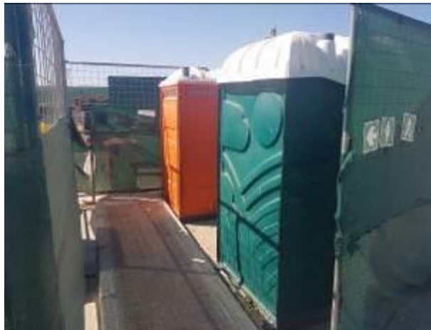
Image 5: Ablutions on site, in working order.
